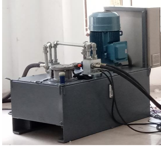
Hydraulic power pack
