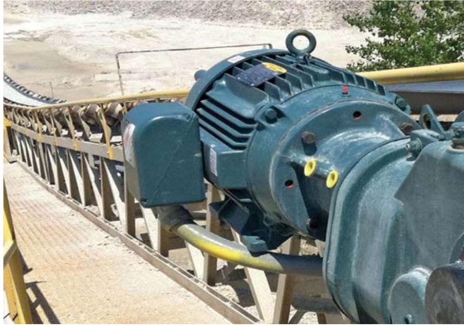
Figure 1.3 Drives in conveyor belts
