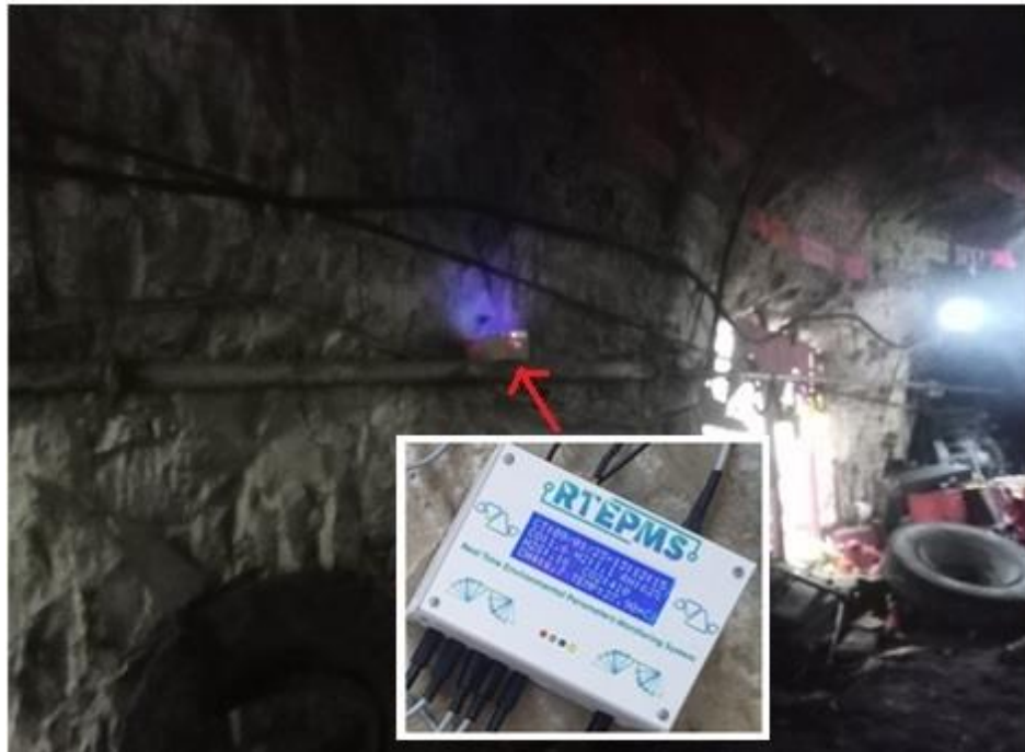
Fig. 5.26 RTEPMS with LoRa transmitter deployment at tunnel 26 of the underground mine 'B'
