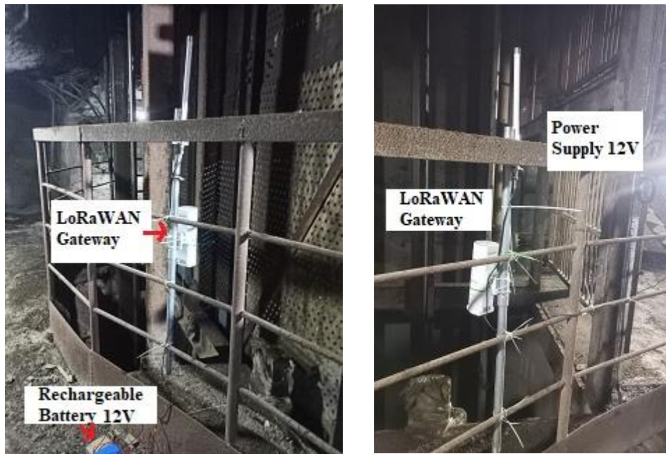
Fig. 5.43 Installation of LoRaWAN Gateway device
