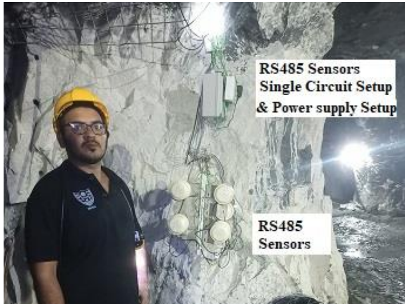
Fig. 5.41 Installation of Multiple RS485 Sensor Node and Connection to RS485-LN device
