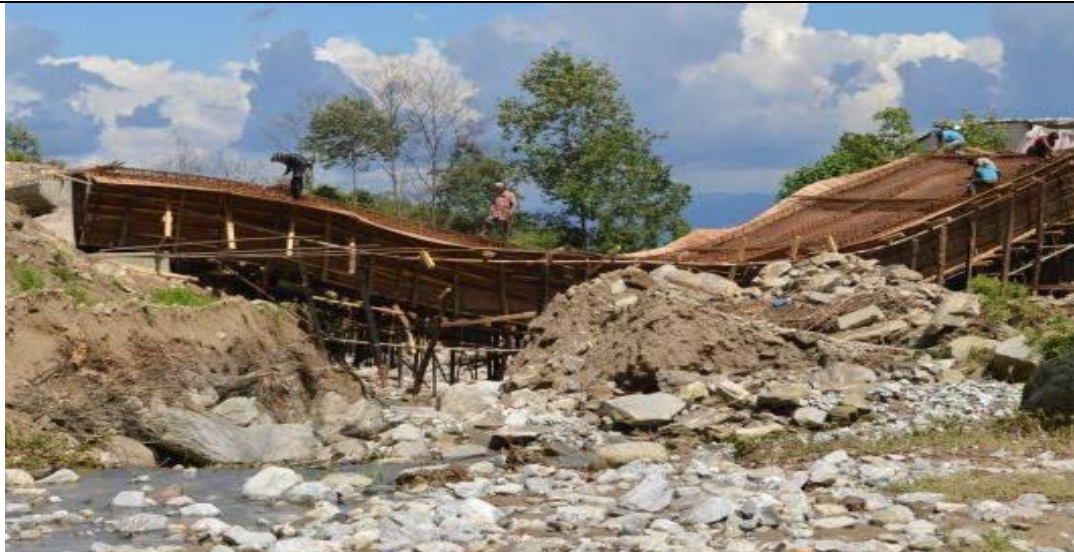
Fig.2 Bridge failure (Infrastructural Damage)
