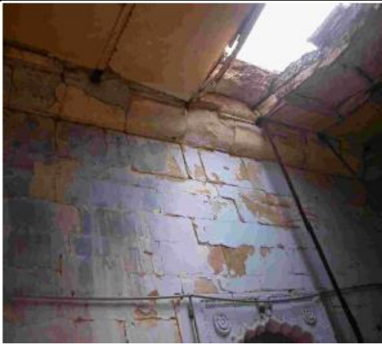
Fig.7 Separation of joist flanges and failure of stone slab (Shethi A et al 2004)
