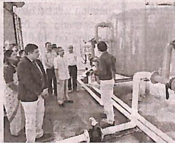
Officials examine the water disinfection plant at NITK, Surathkal | EXPRESS
