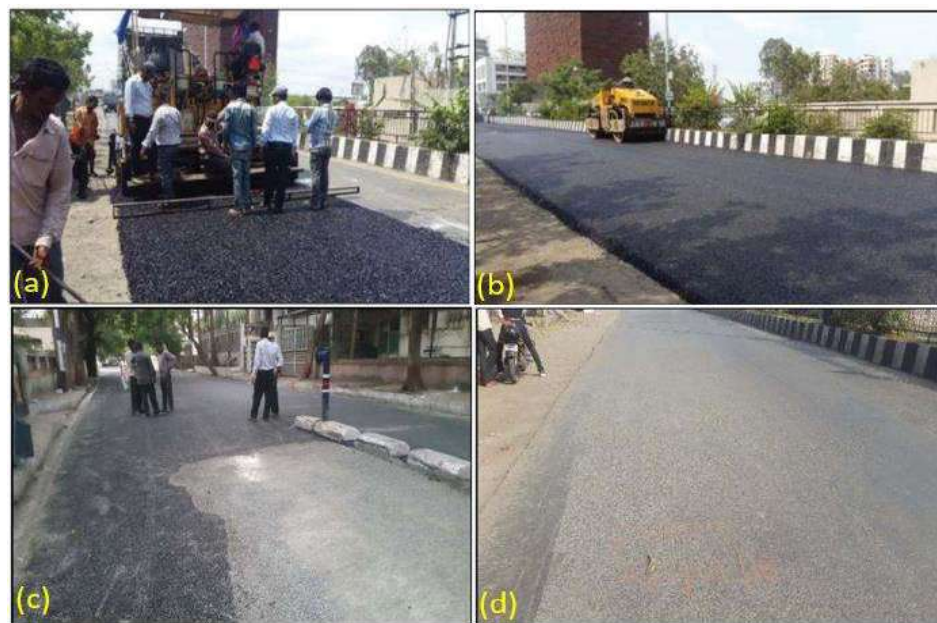
Fig. 1.3 (a) Laying OGA mixture (b) Compaction of OGA mixture (c) Grout poured on OGA layer (d) Finished SFA mixture layer (Bharath et al. 2020)
