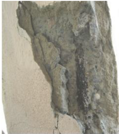
Fig.6.5: View of corroded rebar
