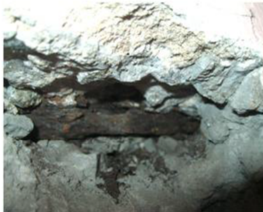
Fig.6.1: Corroded rebar inside beam
